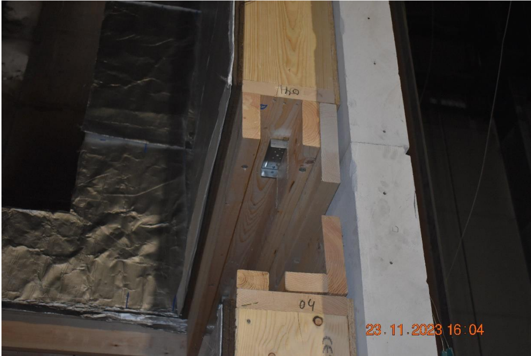
Photo No. 3 Gap between two cassettes.
