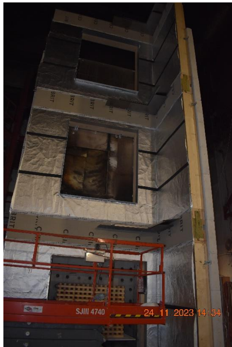
Photo No. 8 FRONT BAND UV 210 tape to tape the overlaps of the membrane.
